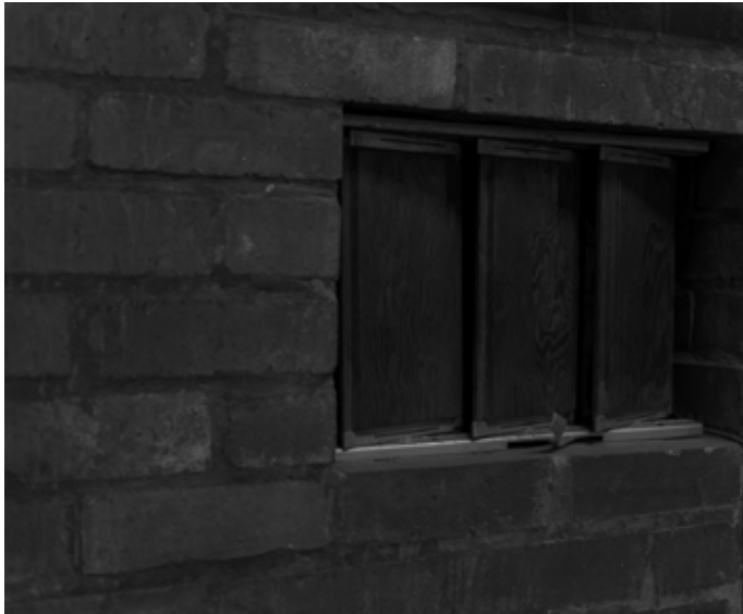
Figure 13 The ingress of fresh air inside the auditorium is controlled by adjustable vertical timber louvre blades at pew height (photo: Roger Jardine).
