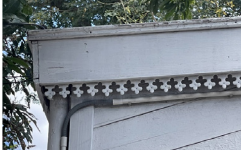
Figure 8 Details of the rainwater drip around the perimeter of the room. An example of ornate lace fascia. (photograph by the author, 2024).
